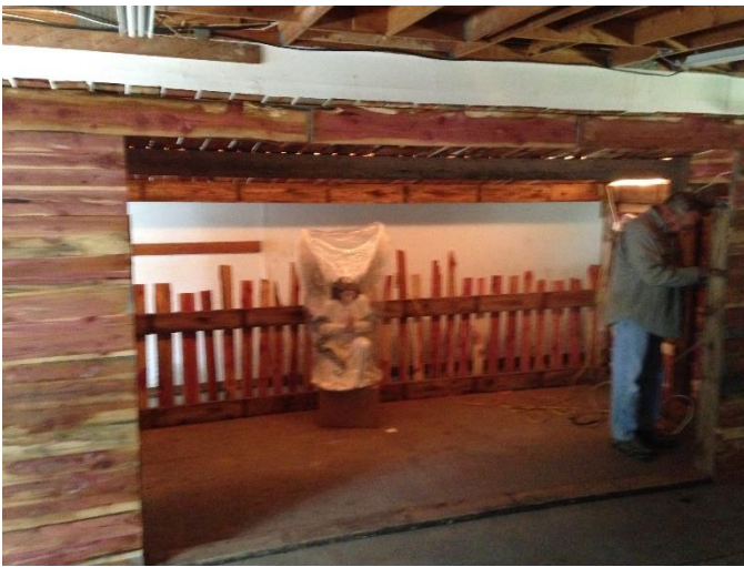
Stable for the new Nativity Scene is ready to go, thanks to our carpenters.
